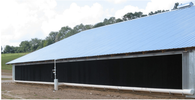
Recirculating Evaporative Cooling System
